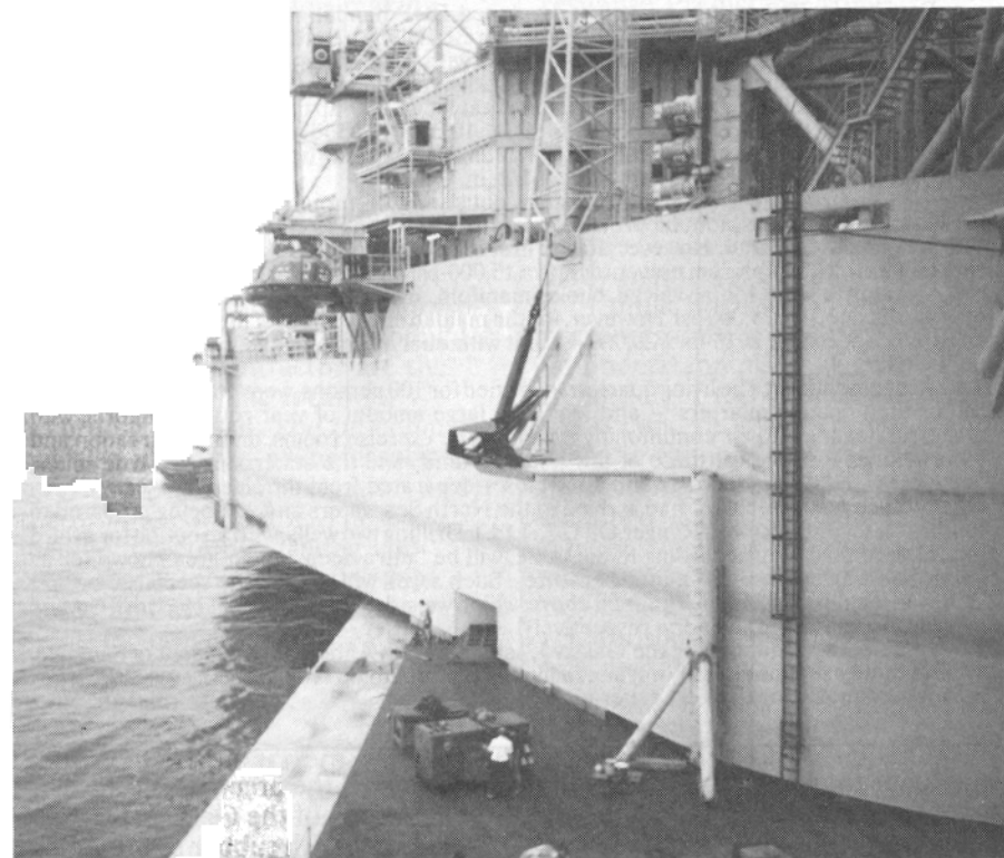
Top: Soft wooden cribbing on the cargo deck of the Transshelf transport vessel, matching the rig's hull framing, was used to transfer static and dynamic loads to the vessel. Above: Partial view of the Galaxy I already sitting on deck. Notice, at left, one of the sponsons.
